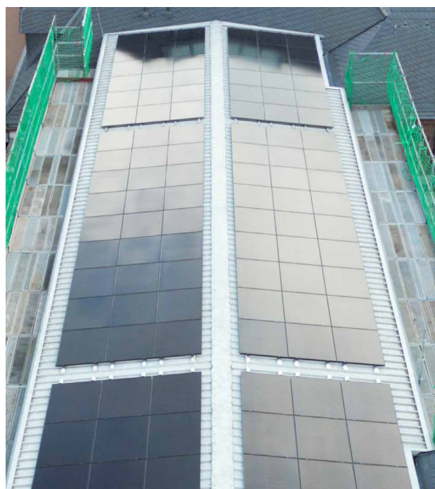
50 kWp solar system at the Haag-Streit Mannheim site
